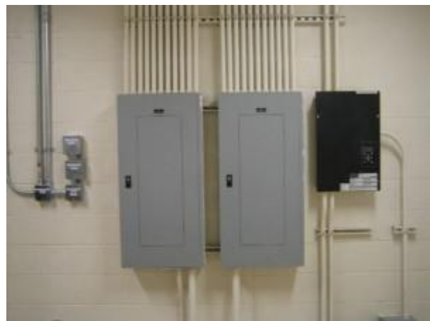
Service drops will create high field on opposing
